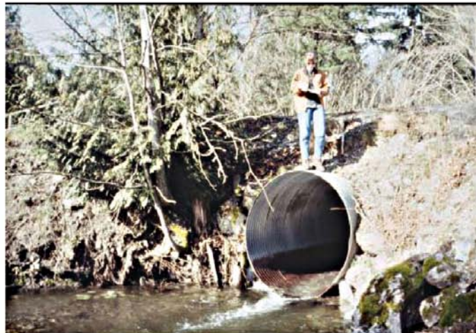
The old crossing was a 6.2 ft (1.89 m) diameter corrugated steel pipe that was a barrier to fish passage due to excessive slope.
