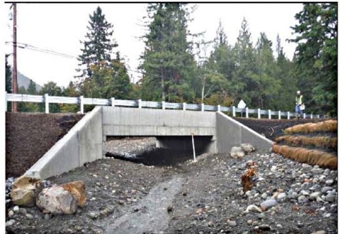
The new crossing is a 27 ft (8.23 m) wide concrete box structure that provides access to 2.4 mi (3.9 km) of potential habitat for chum and coho salmon, steelhead, sea run cutthroat, resident and bull trout.
